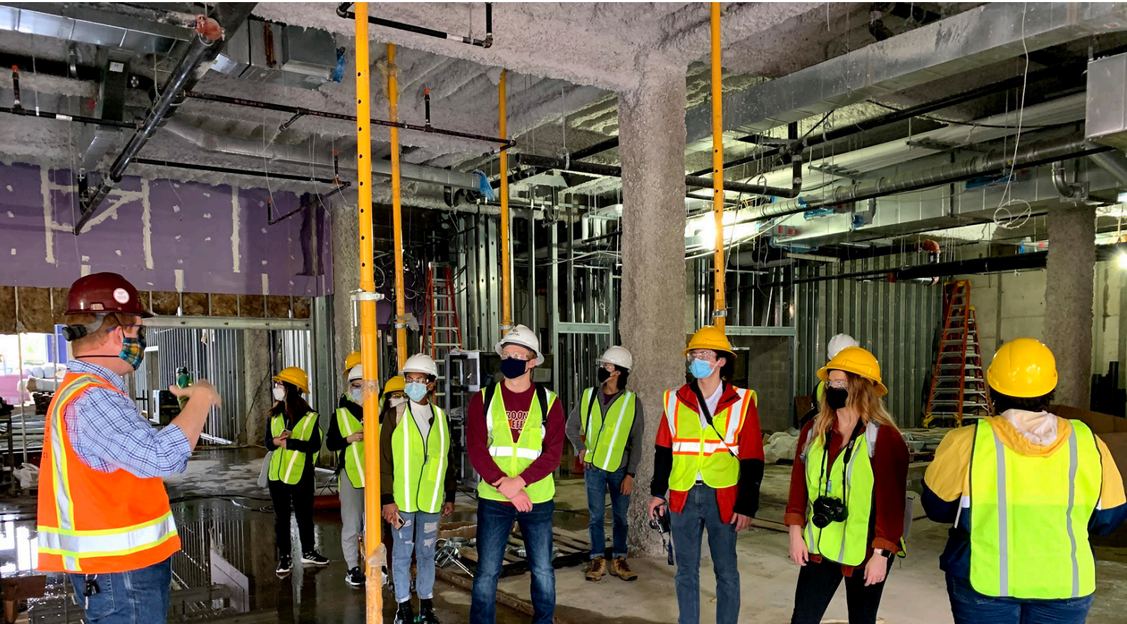
Living Lab #5 Creativity + Innovation District LLC. October 2021. Professor Edward Becker's students visiting the Makerspace at Creativity + Innovation District LLC construction site.
